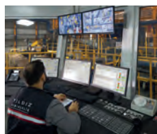
Danieli Automation supplied all of the electrical and control systems
