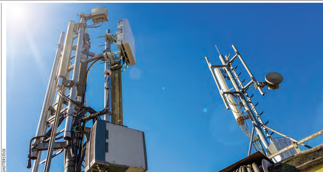
5G smart mobile telephone radio network antenna base station on telecommunication masts
